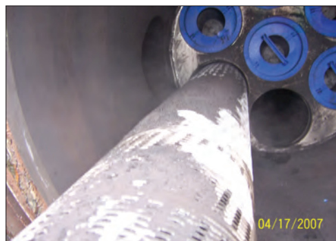
Fig.3. Black powder plugging gas filters.
