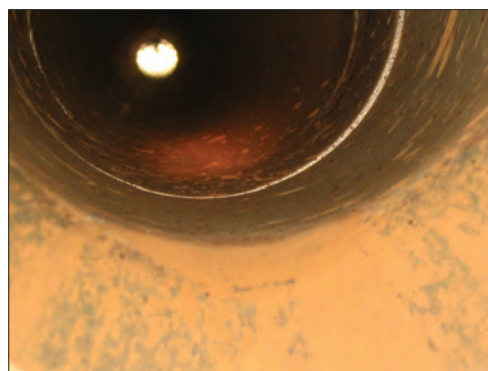
Fig.4. Rouge, finely divided hematite or red rust, is found in a new pipeline left exposed to air. Rouge is a polishing compound and is highly abrasive in pipelines. Rouge will not form in natural gas pipelines due to the low oxygen content of natural gas. Large particle sized hematite is coloured black and can be differentiated from millscale because it is not magnetic.
